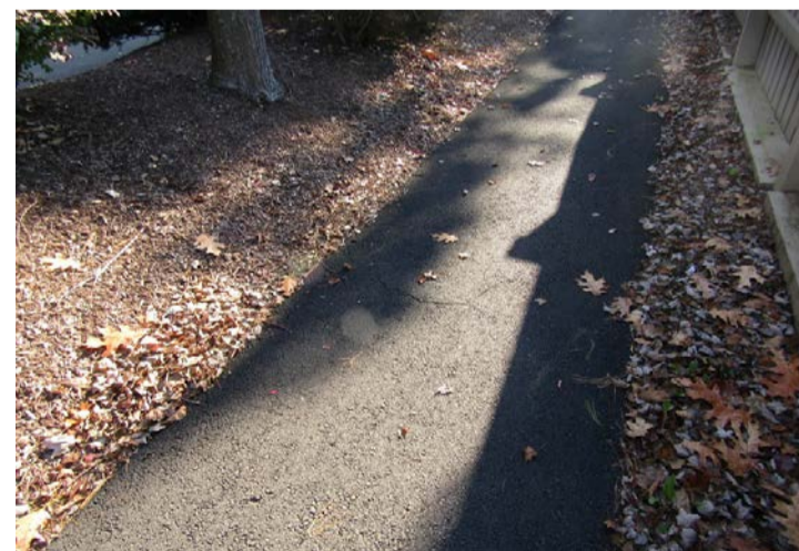
minor crack in newer pavement at tree roots
