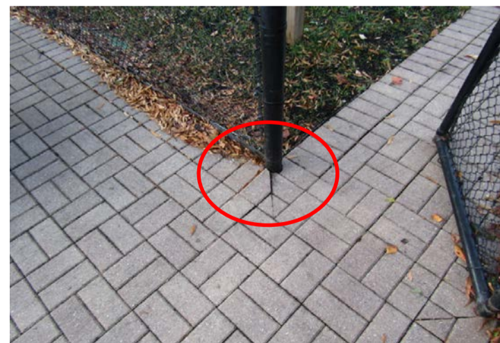
isolated trip hazard
