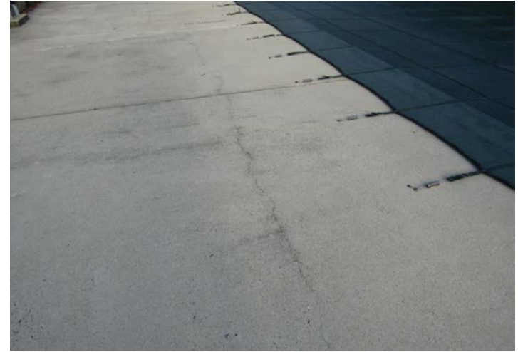
minor cracks in concrete
