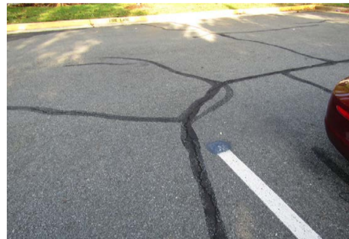
open joints at crack repairs
