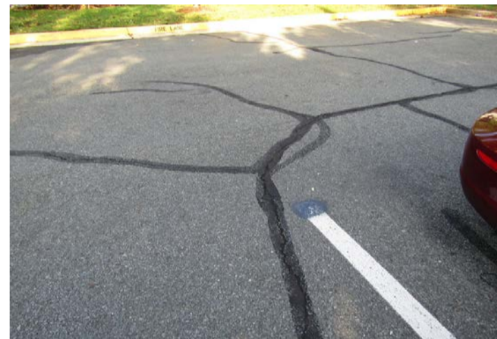
open joints at crack repairs
