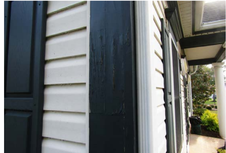
wood trim with peeling paint
