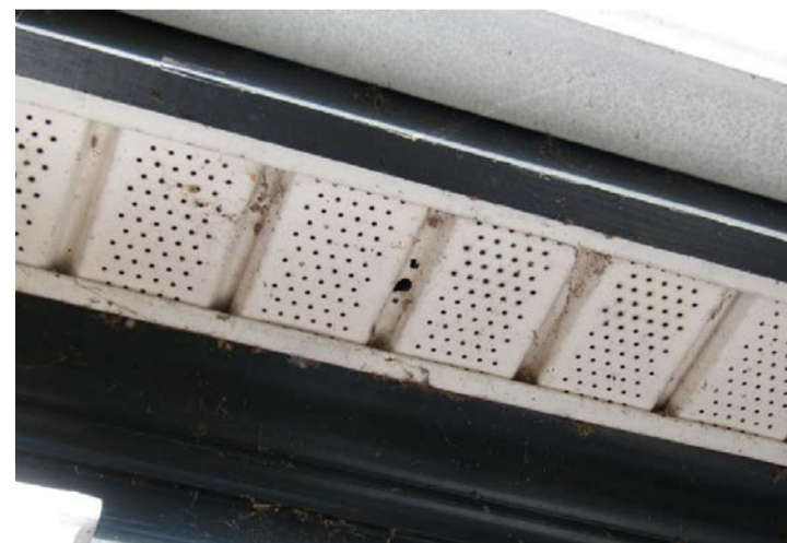
deterioration of soffit
