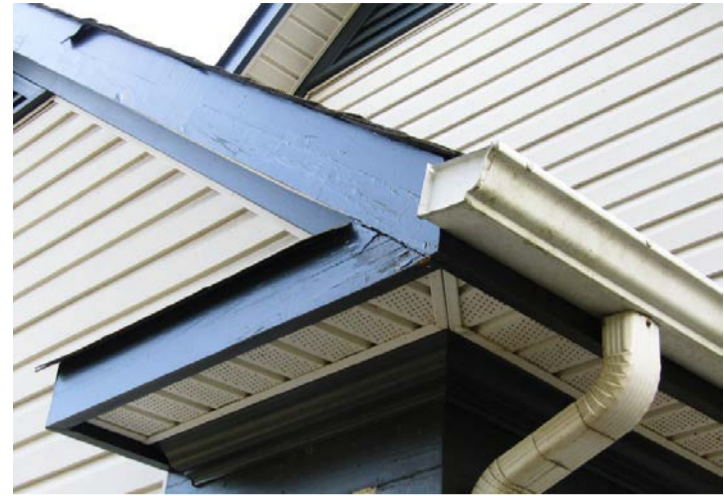
wood trim with deterioration
