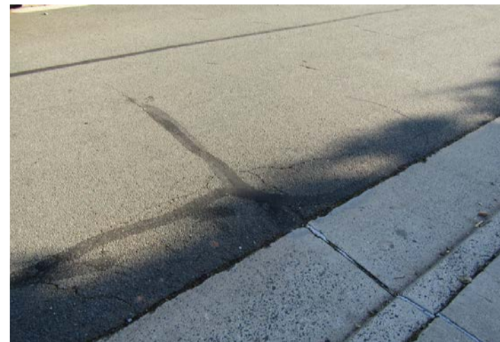
repaired and unrepaired cracks
