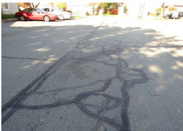
repaired and unrepaired cracks
