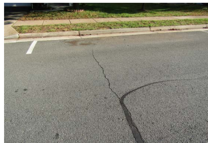
repaired and unrepaired cracks
