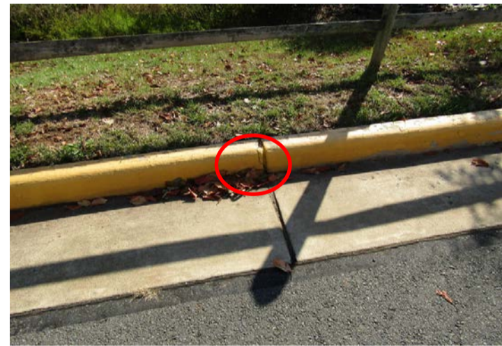
very minor crack near joint
