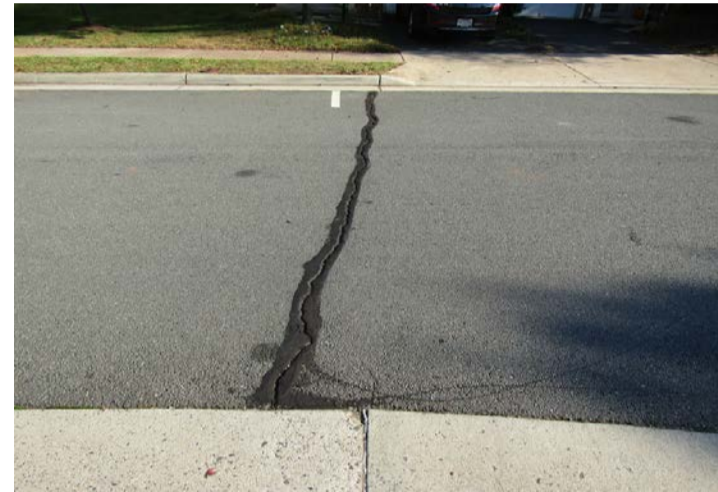
open joint in repaired crack
