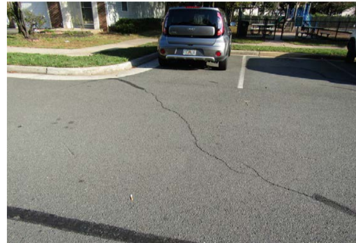
repaired and unrepaired cracks
