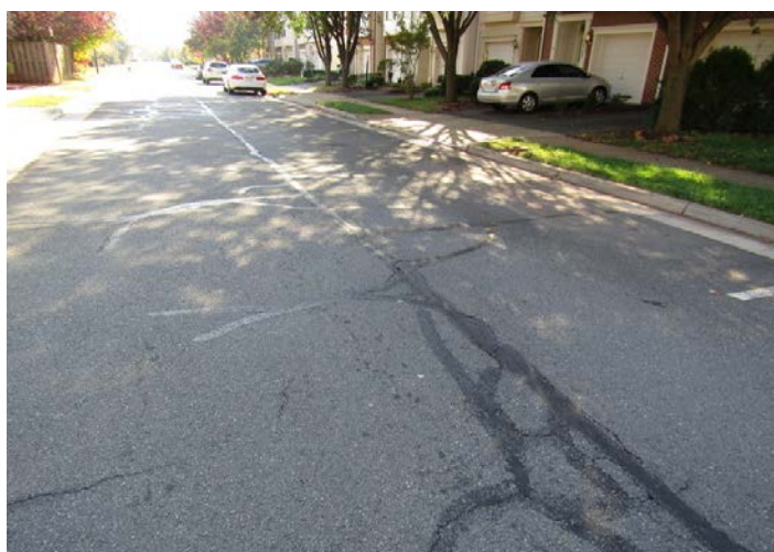
crack repairs and deterioration
