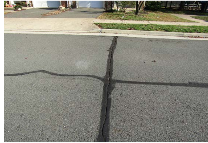
open joint in repaired crack
