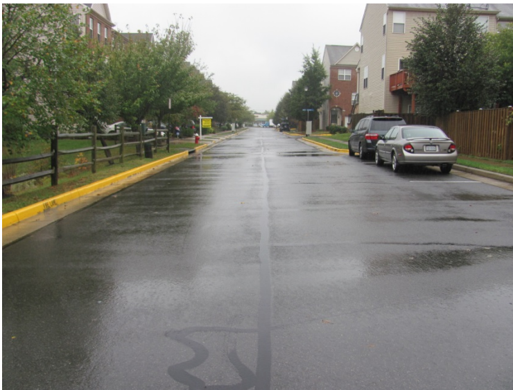
Townhome asphalt pavement cracks and crack repair
