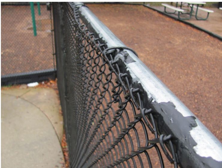
Chain link fence vinyl coating deterioration
