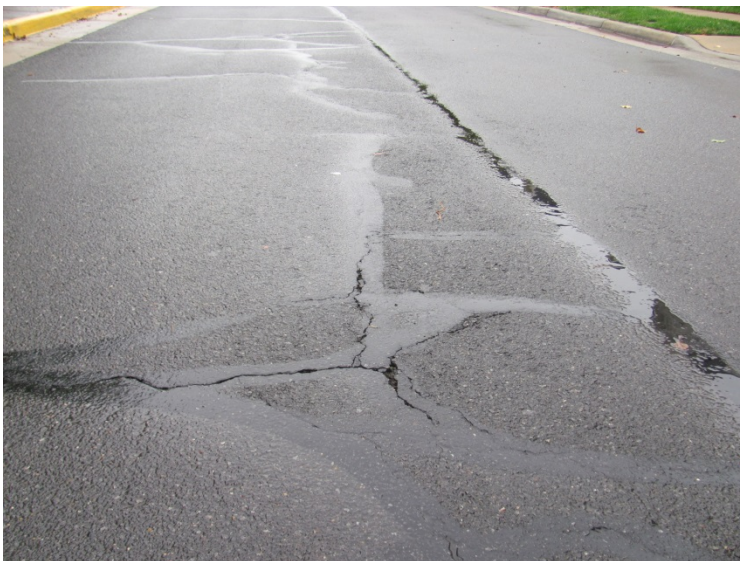
Townhome asphalt pavement cracks and crack repair
