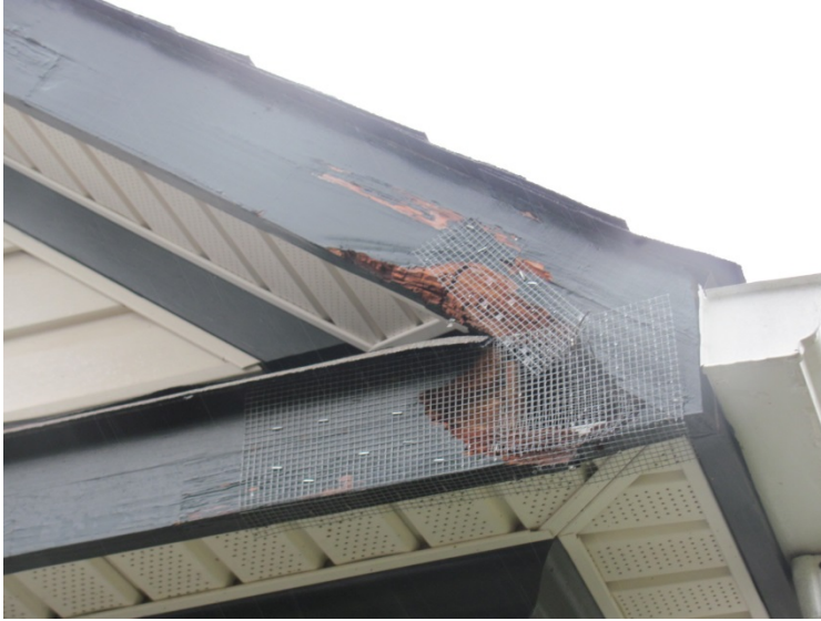
Pool house exterior wood trim deterioration
