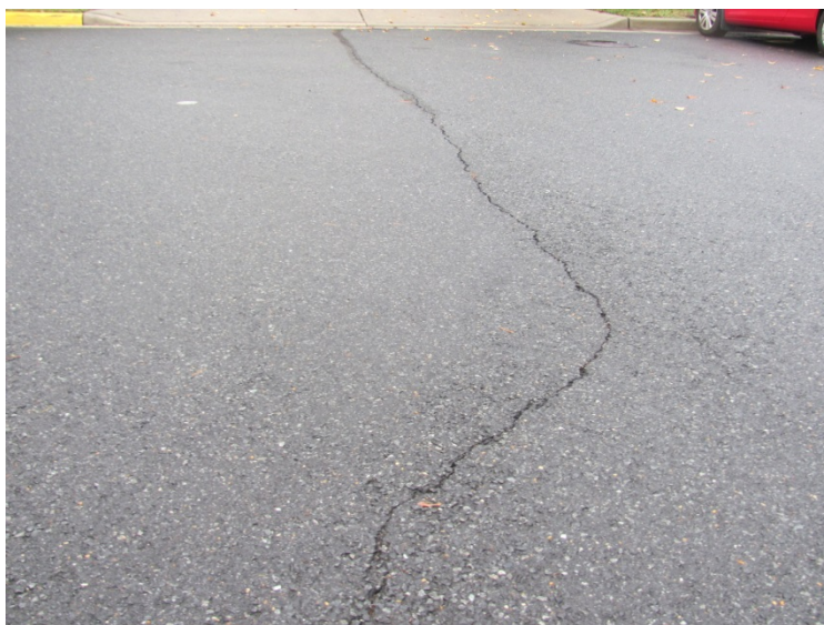
Townhome asphalt pavement cracks
