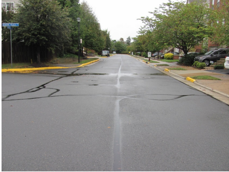
Townhome asphalt pavement cracks and crack repair
