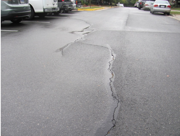
Townhome asphalt pavement cracks and crack repair
