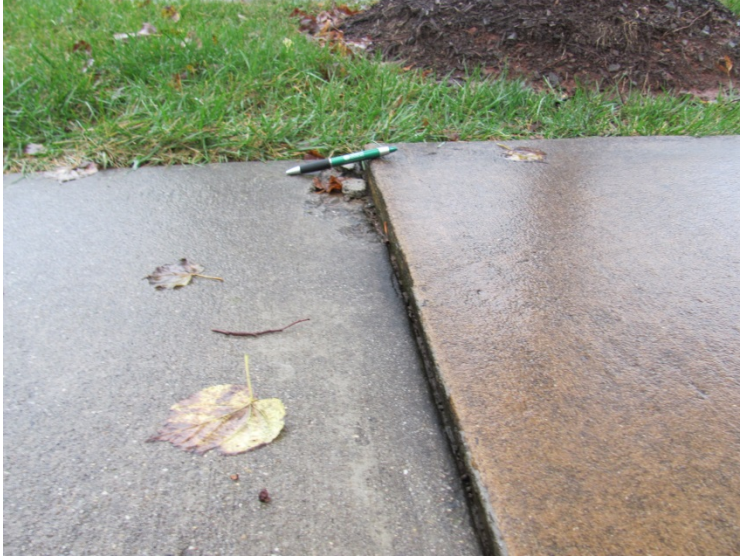
Townhome concrete sidewalk settlement
