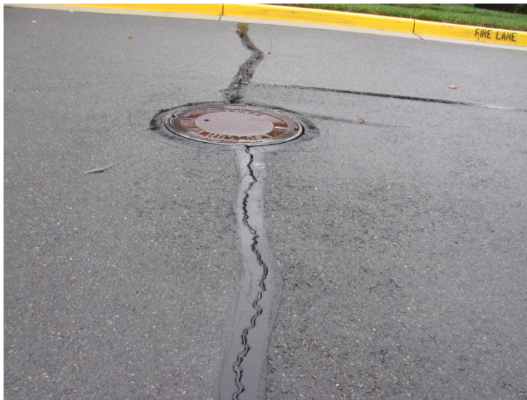
Townhome asphalt pavement cracks and crack repair
