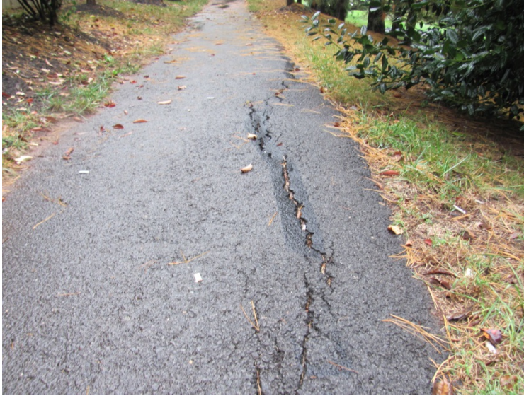
Asphalt pavement walking path edge cracks parallel to Southern Oaks Terrace
