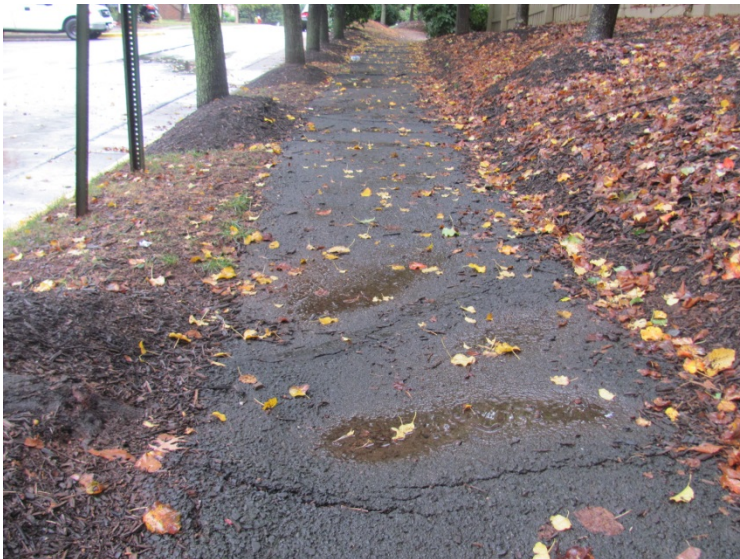
Asphalt pavement walking path tree root damage parallel to Southern Oaks Terrace
