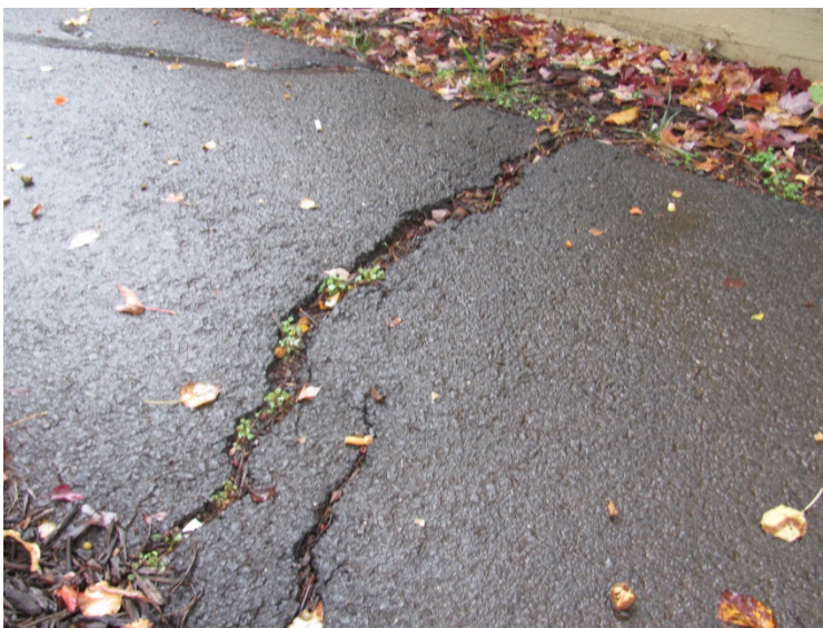
Asphalt pavement walking path cracks parallel to Southern Oaks Terrace
